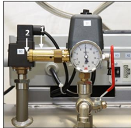
Fig. 25: Check of safety valve
