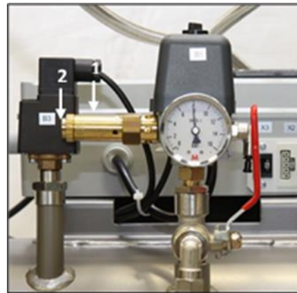
Fig. 25: Check of safety valve
