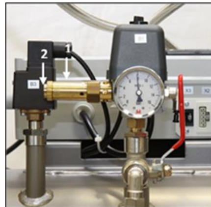
Fig. 25: Check of safety valve
