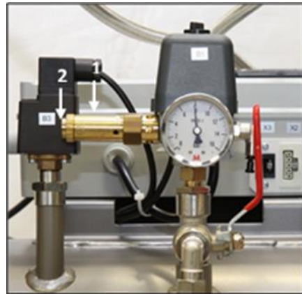
Fig. 17: Check of safety valve
