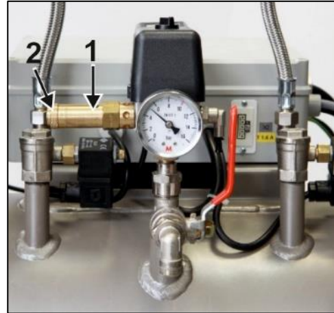
Fig. 24: Check of safety valve
