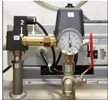
Fig. 17: Check of safety valve
