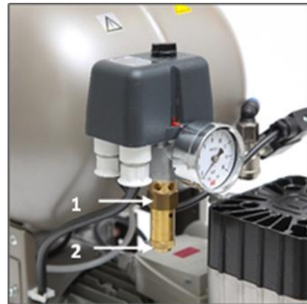
Fig. 7: Check of safety valve
